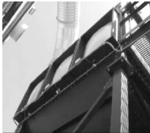
Figure 1. Outdoors Explosion Vent Installation On Dust Collector
